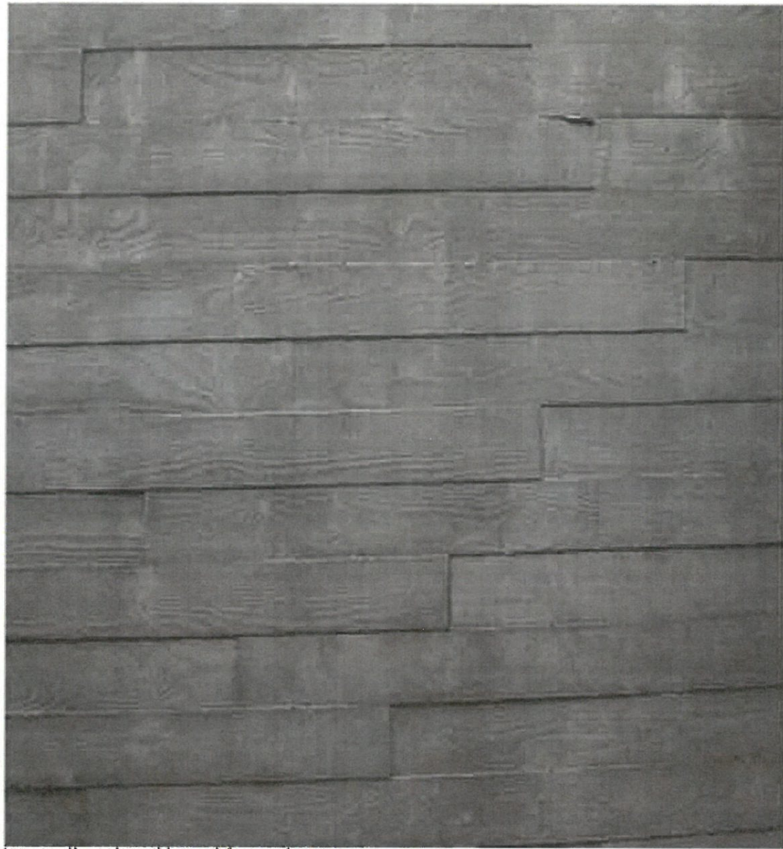
integrally colored board formed concrete
