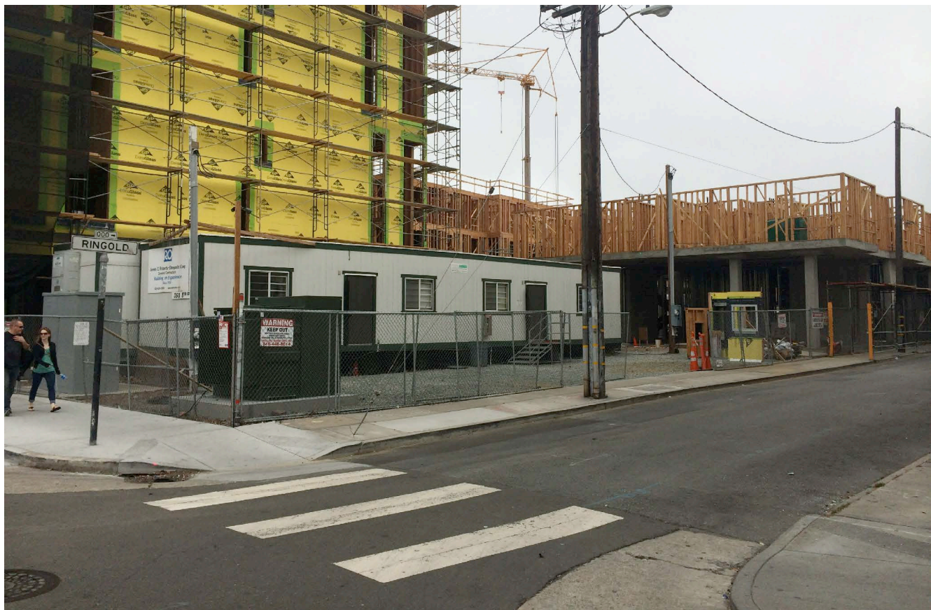
1 RINGOLD ALLEY @ 8TH STREET - SE CORNER SITE OF NEW PARK & PROPOSED FEATURE CROSSWALK
