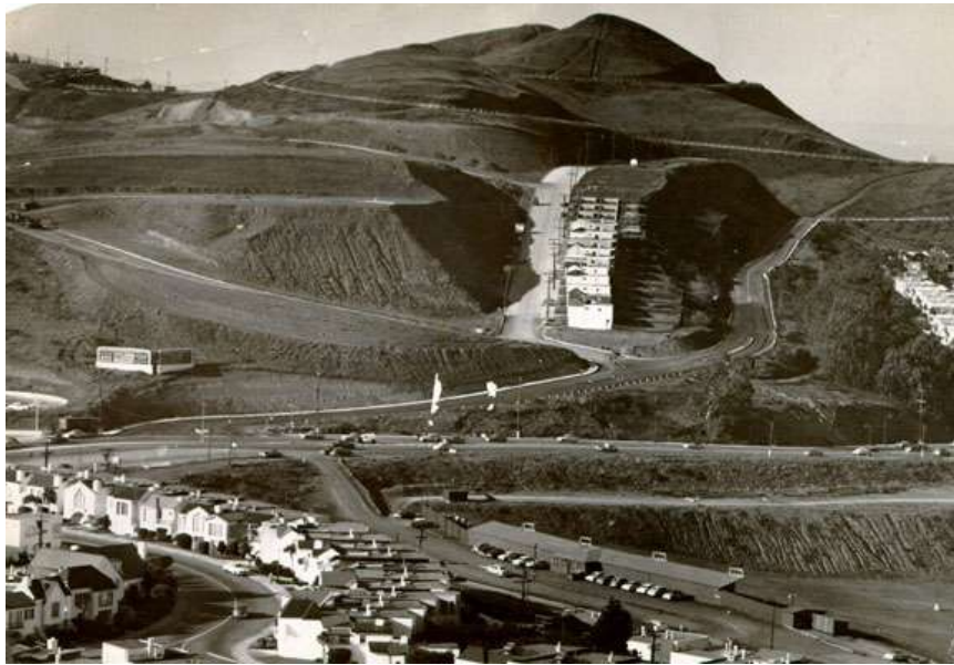
(Photo of the extensive grading and shoring undertaken for a new development to become the Midtown Terrace / Forest Knolls neighborhoods taken on April 13, 1953.
