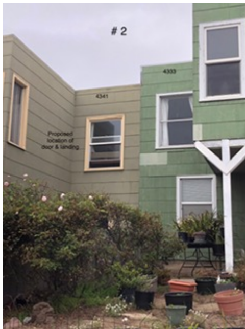
Photo # 2: proposed location for door and landing at 4341 Ulloa Street proposed location for rear stair deck at 4341 Ulloa Street
