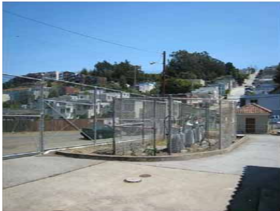
View of PG&E Transformer Equipment
