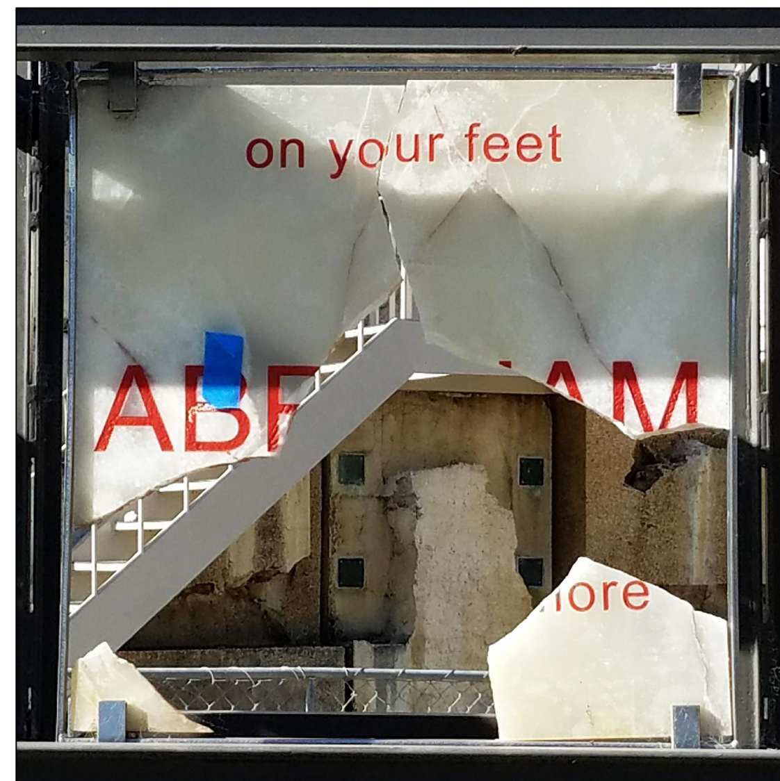
4 DAMAGED PANEL EXAMPLE, 11/04/2016 A2.1 NOT TO SCALE
