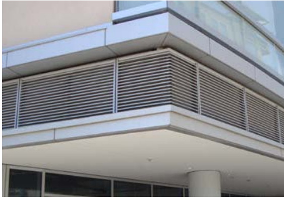
Aluminum Louvers – Lot DD Station
