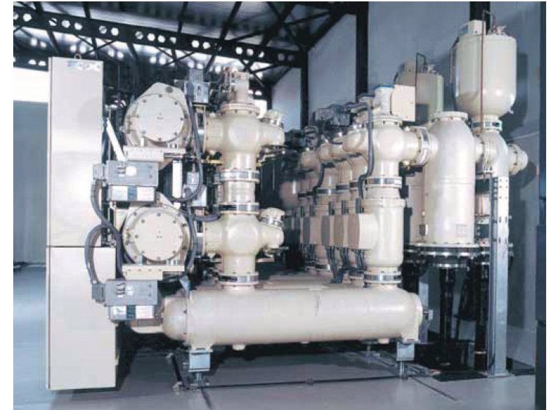
Gas Insulated Switchgear
