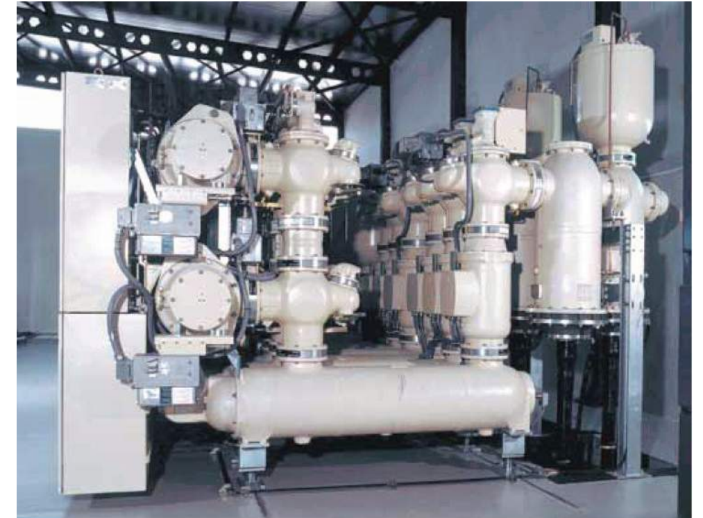
Gas Insulated Switchgear
