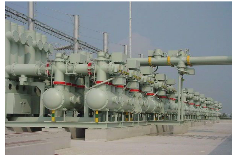
Gas Insulated Switchgear
