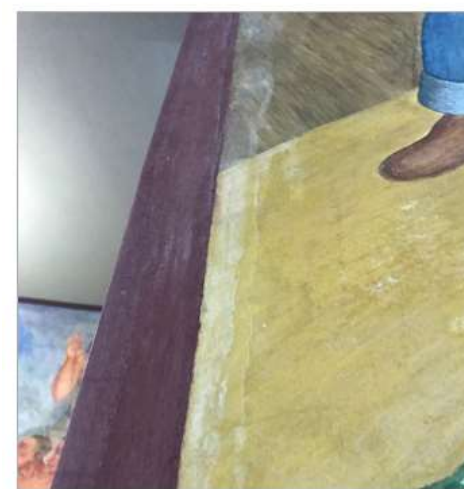
Figure 12: Detail of efflorescence on the Outdoor Life mural. Notice pattern followed by water coming from ceiling.
