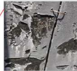
Figure 2: Deteriorated fiberglass roof.
