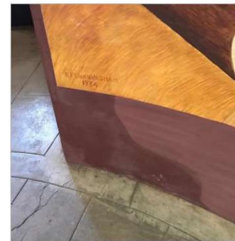
Figure 13: Detail of efflorescence on the Outdoor Life mural. Light accretions were emerging on the wall.
