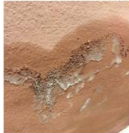
Figure 19: Detail of growing efflorescence at the bottom of the Powell Street mural's stucco frame. Notice wall still looks wet.
