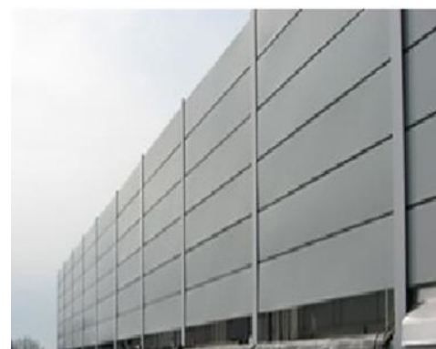
The chiller acoustic screens (Sound Barriers) The color code: Gray, RAL 7040 match with lighter cement plaster.
