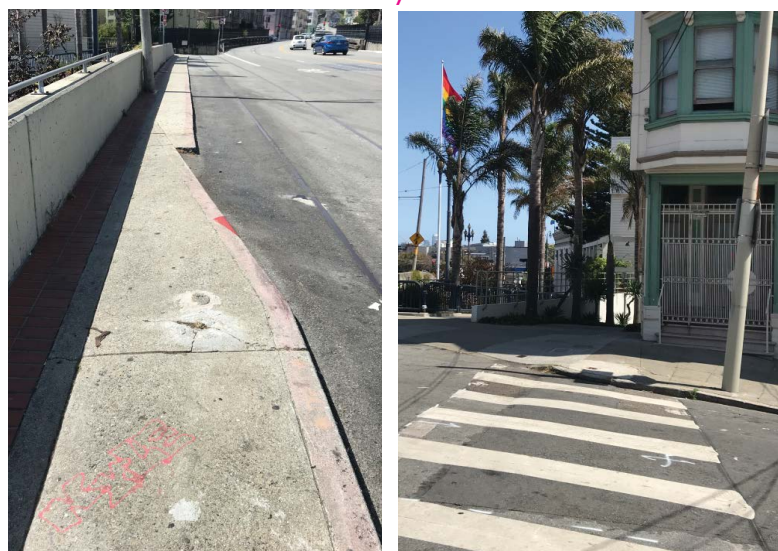
Add new curb ramp at intersection of Market and Collingwood. Widen Market Street Sidewalk east of Collingwood to match width of adjacent sidewalk.
