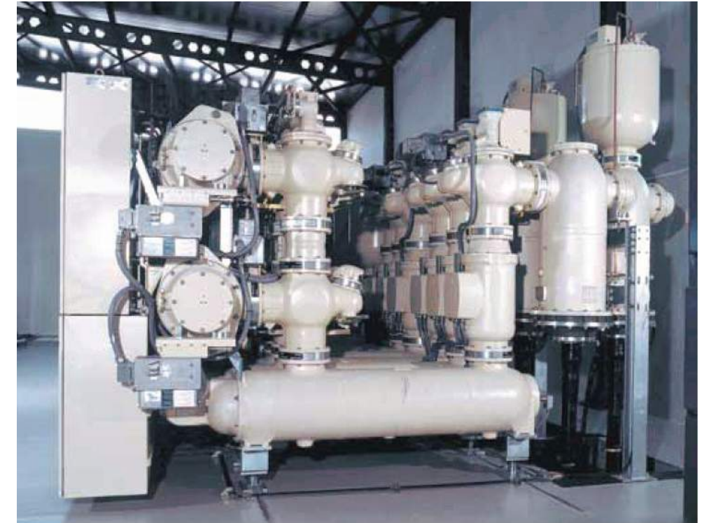
Gas Insulated Switchgear
