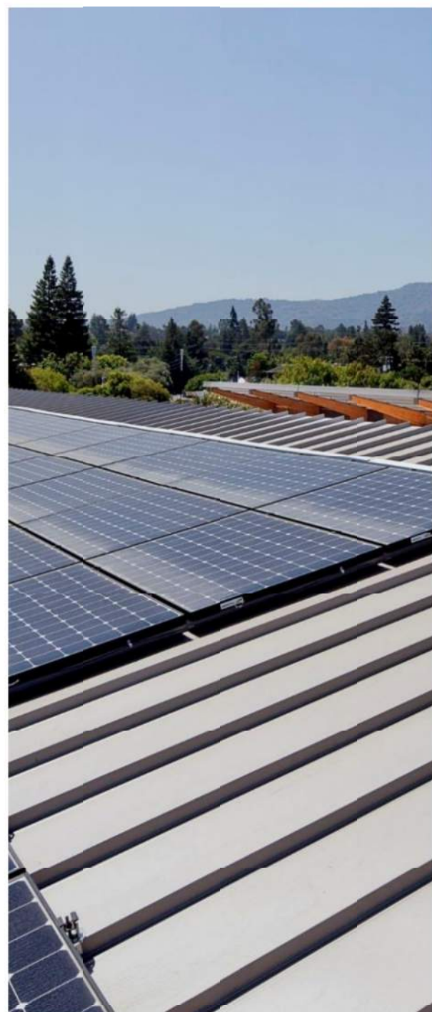
Metal roof with PVs
