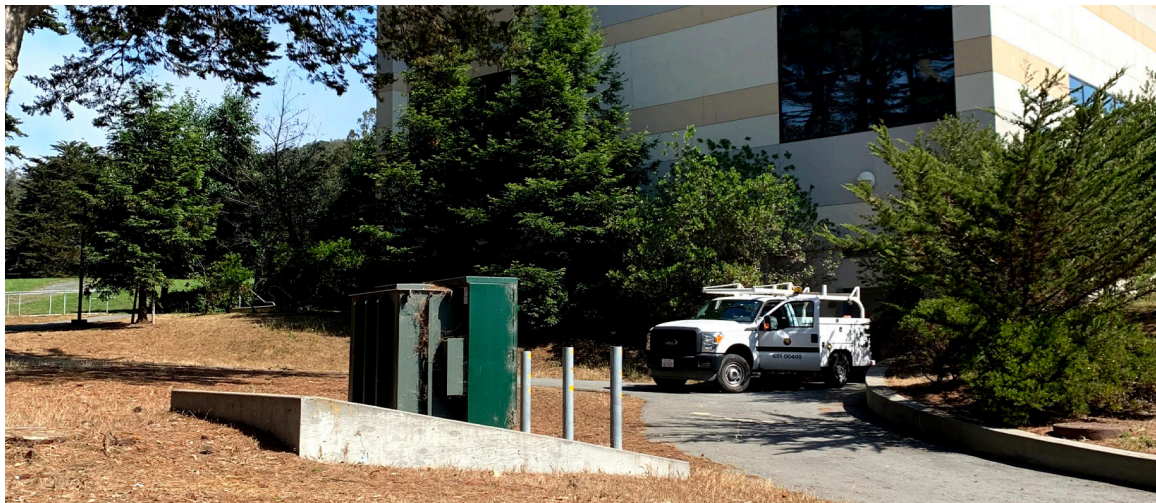
(E) COFFMAN POOL TRANSFORMER AT SOUTH OF BUILDING SITE
