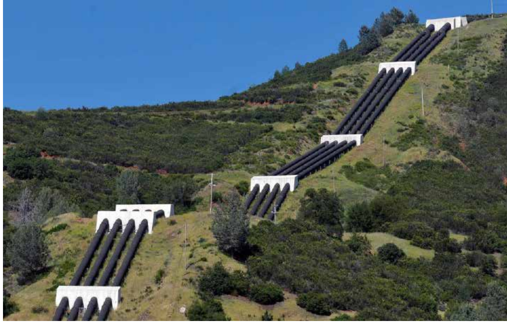
Water being piped in from Hetch Hetchy Reservoir to the New Power Plant
