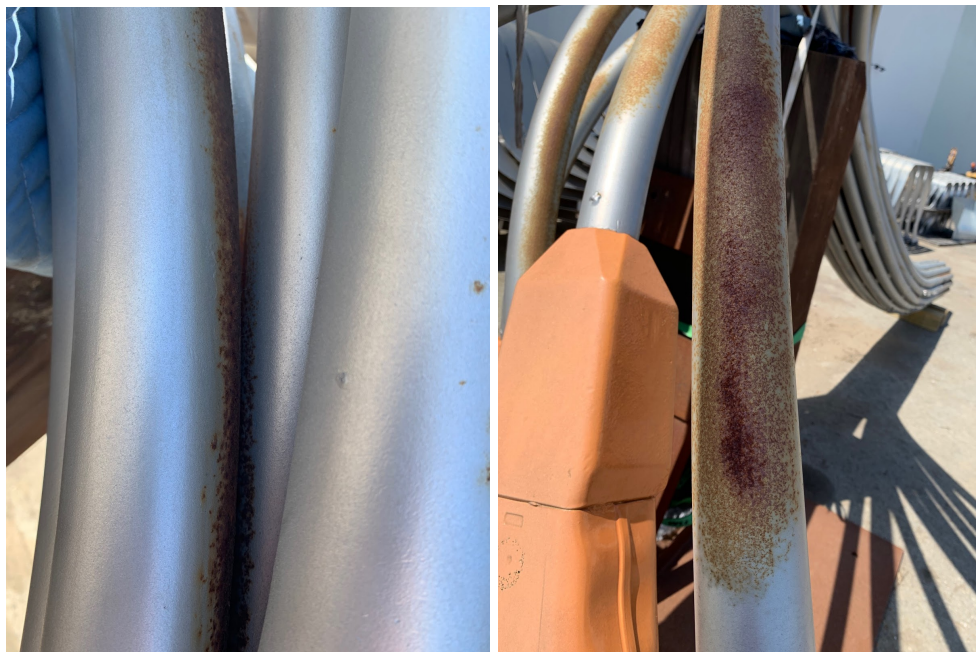
Corrosion on Inaccessible Areas Between Pipes and Upper Surfaces, and Failure of Paint System
