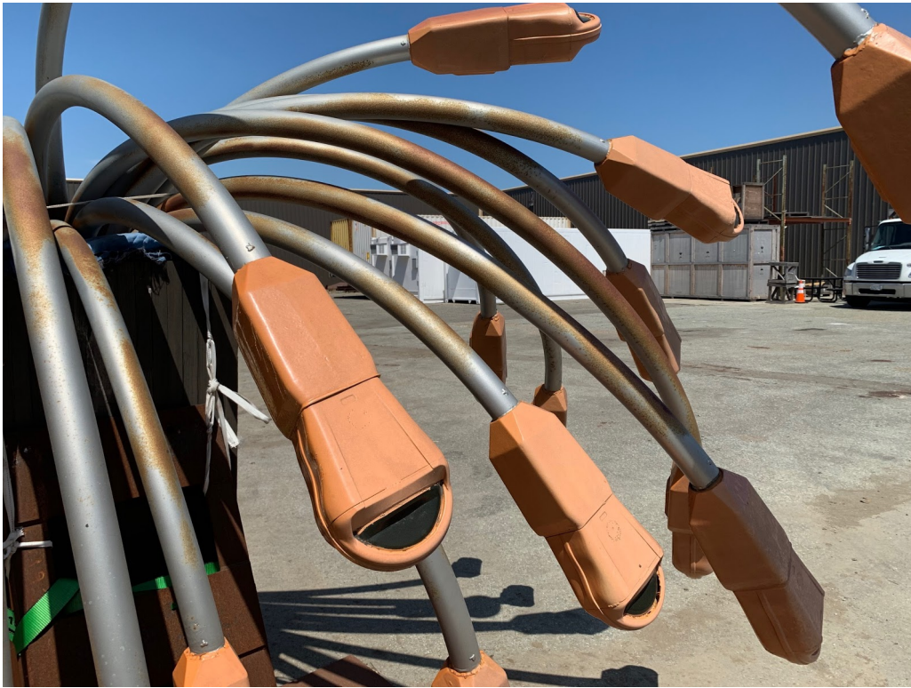
Corrosion on Upper Surfaces of Pipes, and Fading of Orange Paint on Meters
