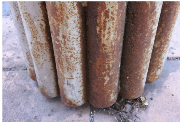
Detail of Corrosion on the Base, Largely from Dog Urine
