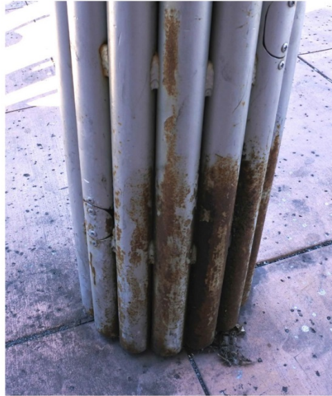
View of the Base, Loss of Coatings and Extensive Ferrous Corrosion
