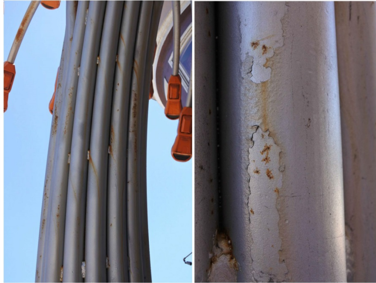
View of Center Section (Left) with corrosion forming along lines of water migration between the pipes Detail of Deterioration of Top Coat Exposing the Primer on Center Section (Right)
