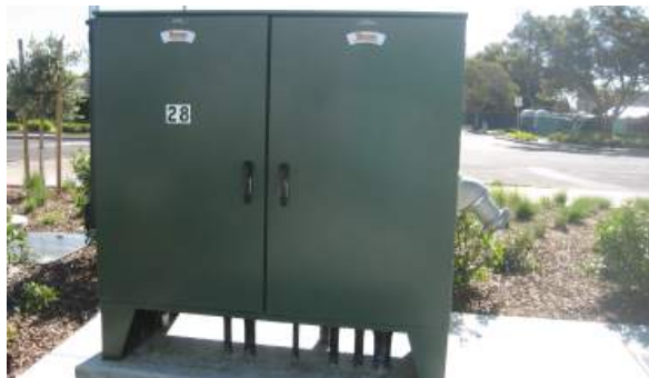
MOTOR CONTROL CENTER
