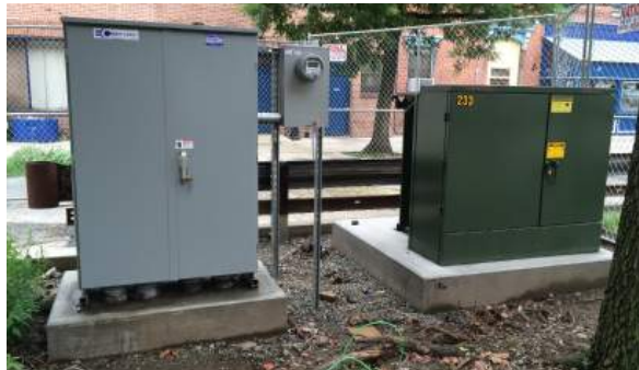
SWITCH BOARD AND TRANSFORMER
