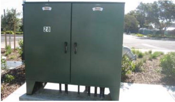
MOTOR CONTROL CENTER
