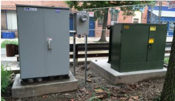
SWITCH BOARD AND TRANSFORMER
