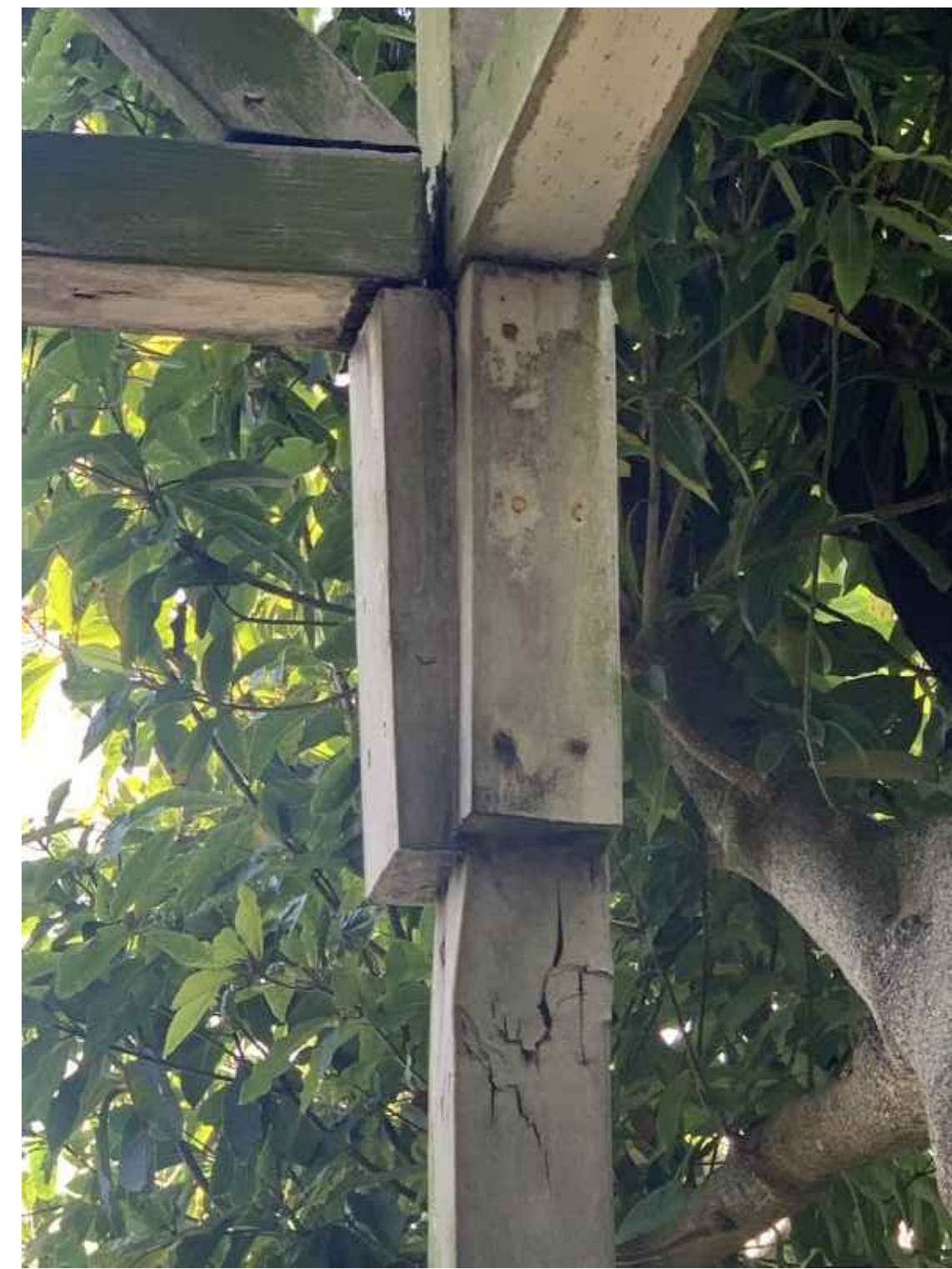
7 TYPICAL DRY-ROTTED POST
