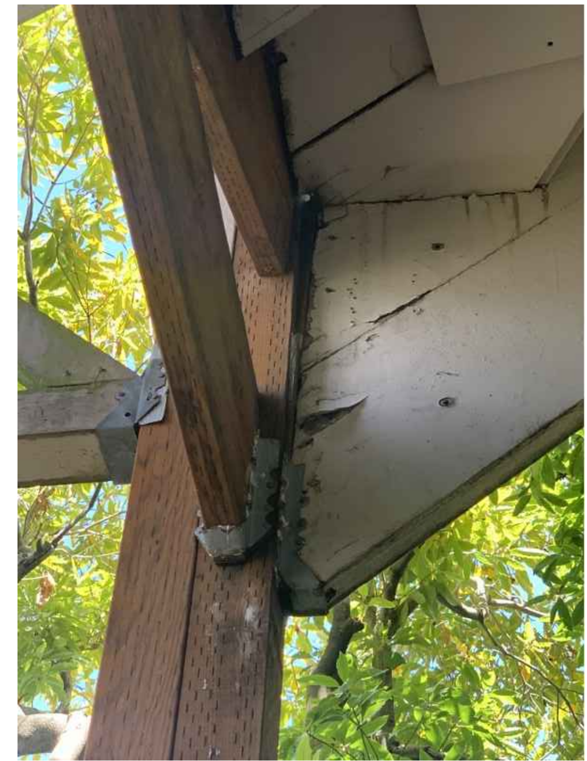
8 TYPICAL DRY-ROTTED STRINGER
