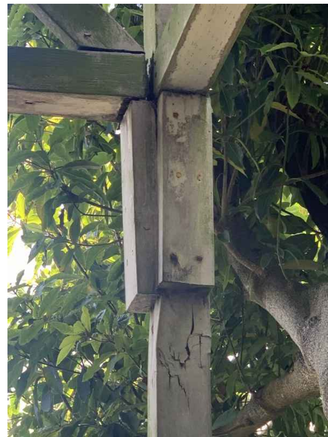
7 TYPICAL DRY-ROTTED POST
