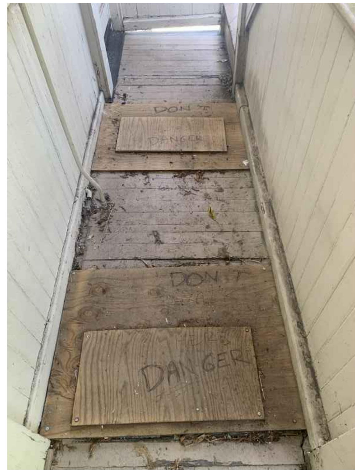
6 TYPICAL DAMAGED SLOPING LANDING
