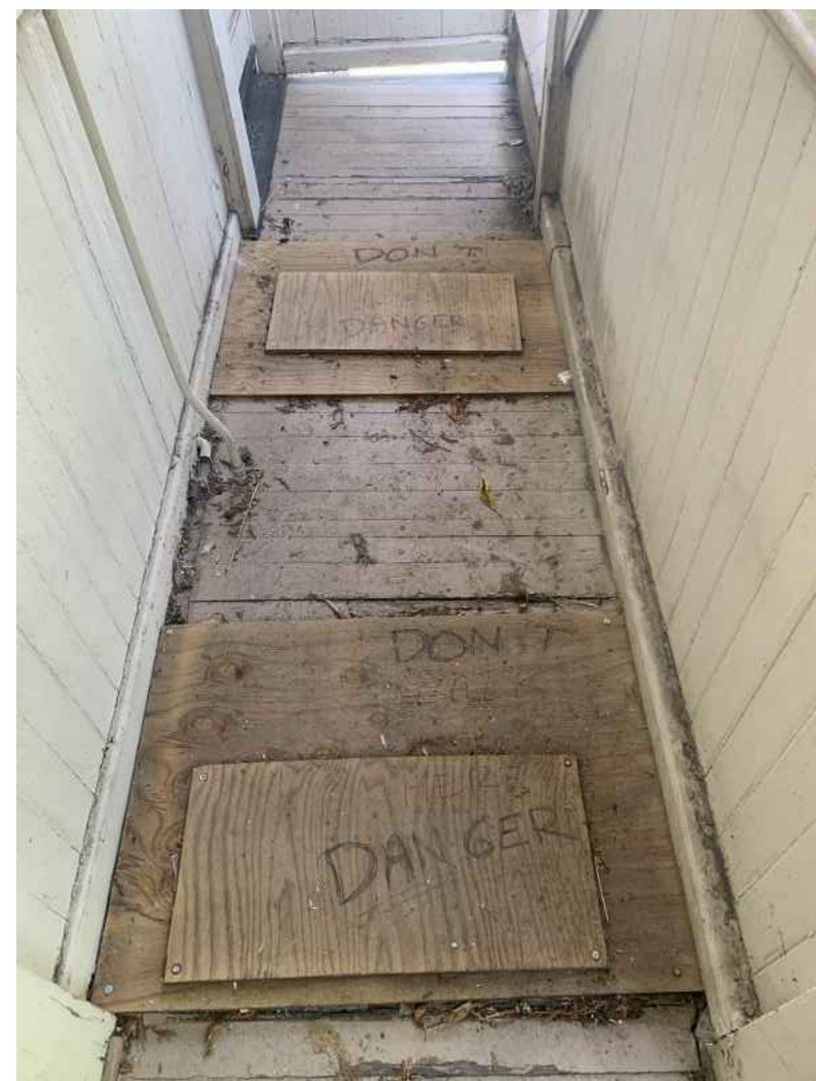
6 TYPICAL DAMAGED SLOPING LANDING
