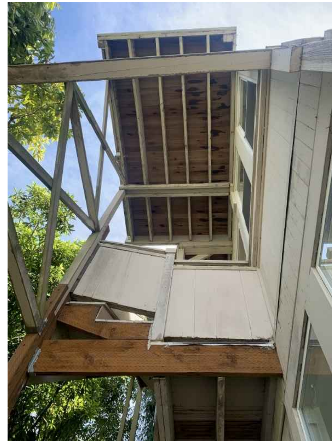
3 (E) 3RD FLOOR DECK TO BE REBUILT
