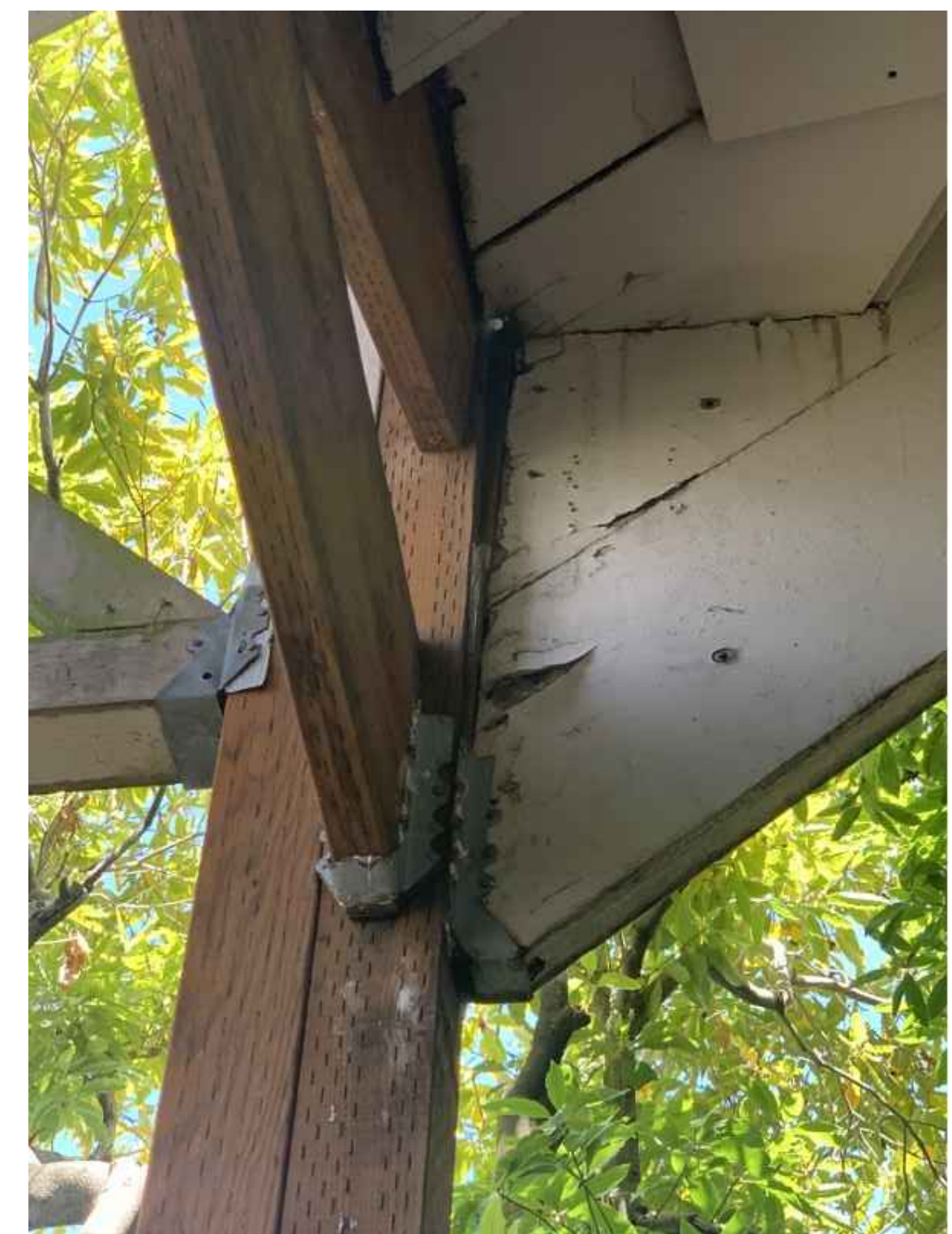
8 TYPICAL DRY-ROTTED STRINGER
