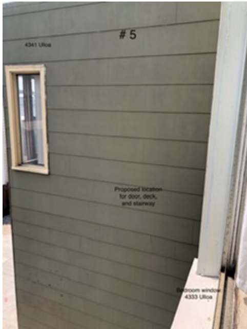
Photo # 5: 4341 Ulloa - proposed location for door, landing, and stairway (taken from upstairs bedroom window at 4333 Ulloa)
