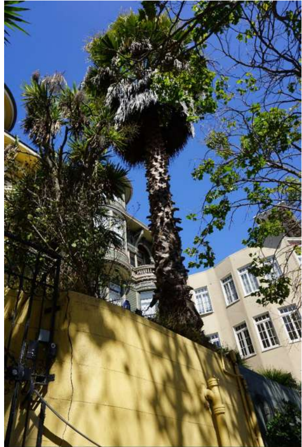
Photo 1 – 40’ tall Mexican fan palm atop a 10’ retaining wall in the front yard.
