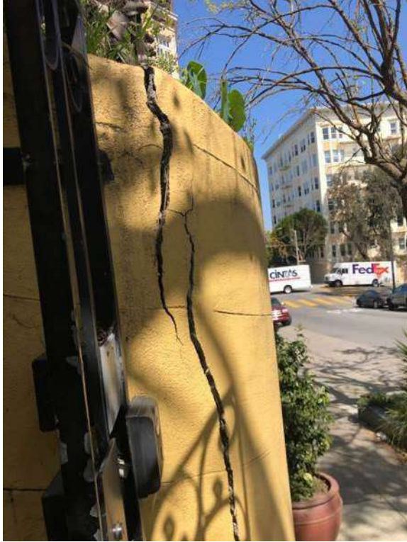
Photo 7 – Cracks in the retaining wall.
