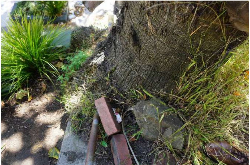
Photo 4 – The overgrown roots in this area dominate the top of the wall that separates the neighbor’s yard.
