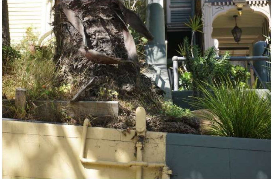
Photo 3 – The palm’s roots are overgrown and exceed the limits of the retaining wall. The palm is being shored by lumber.
