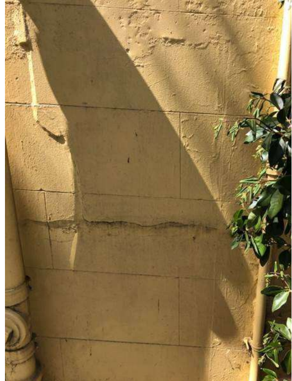
Photo 8 – Cracks in the retaining wall.
