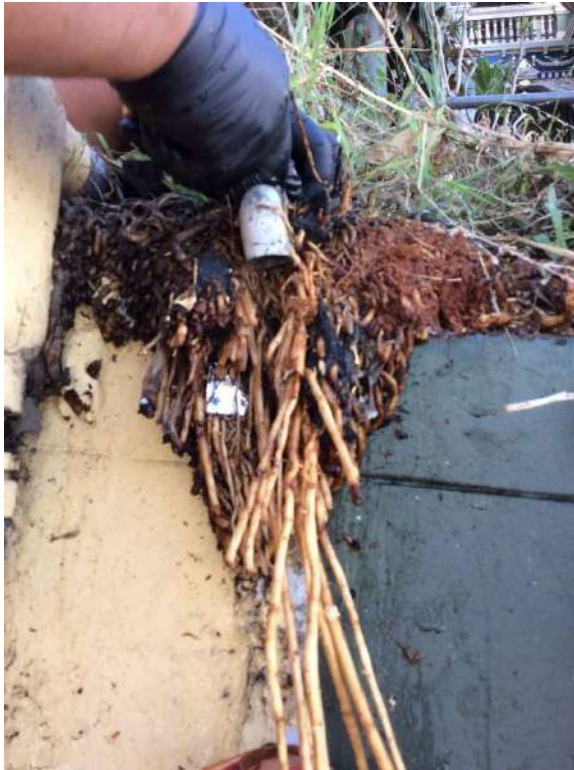
Photo 5 – Palm roots interfering with pipe.
