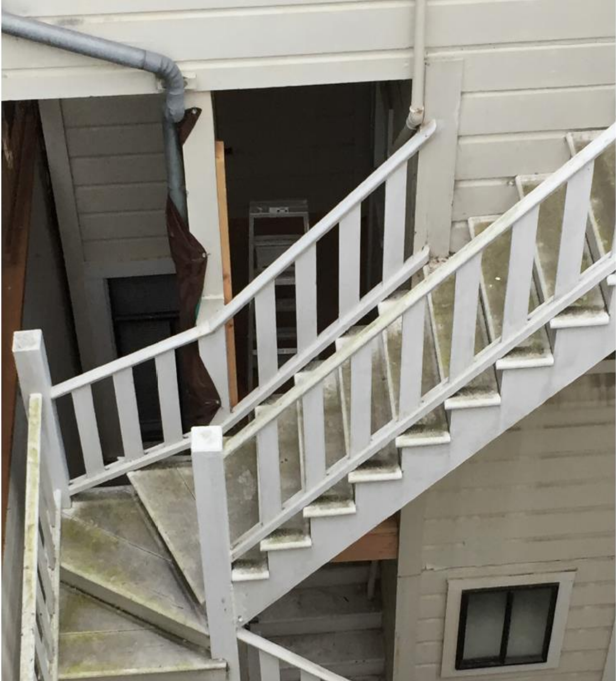
Unpermitted rearward (east) expansion of the first floor
