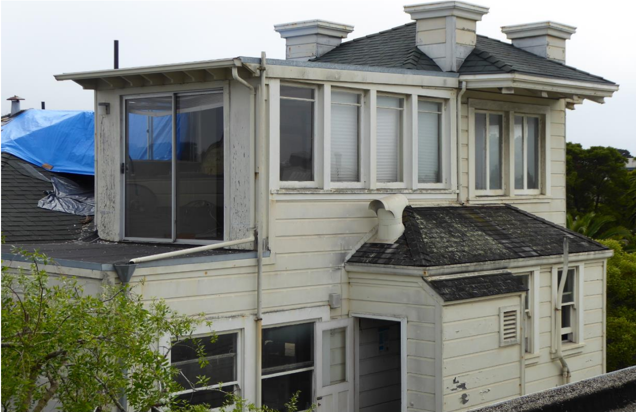
Close up of the penthouse note blue tarp covering framing.
