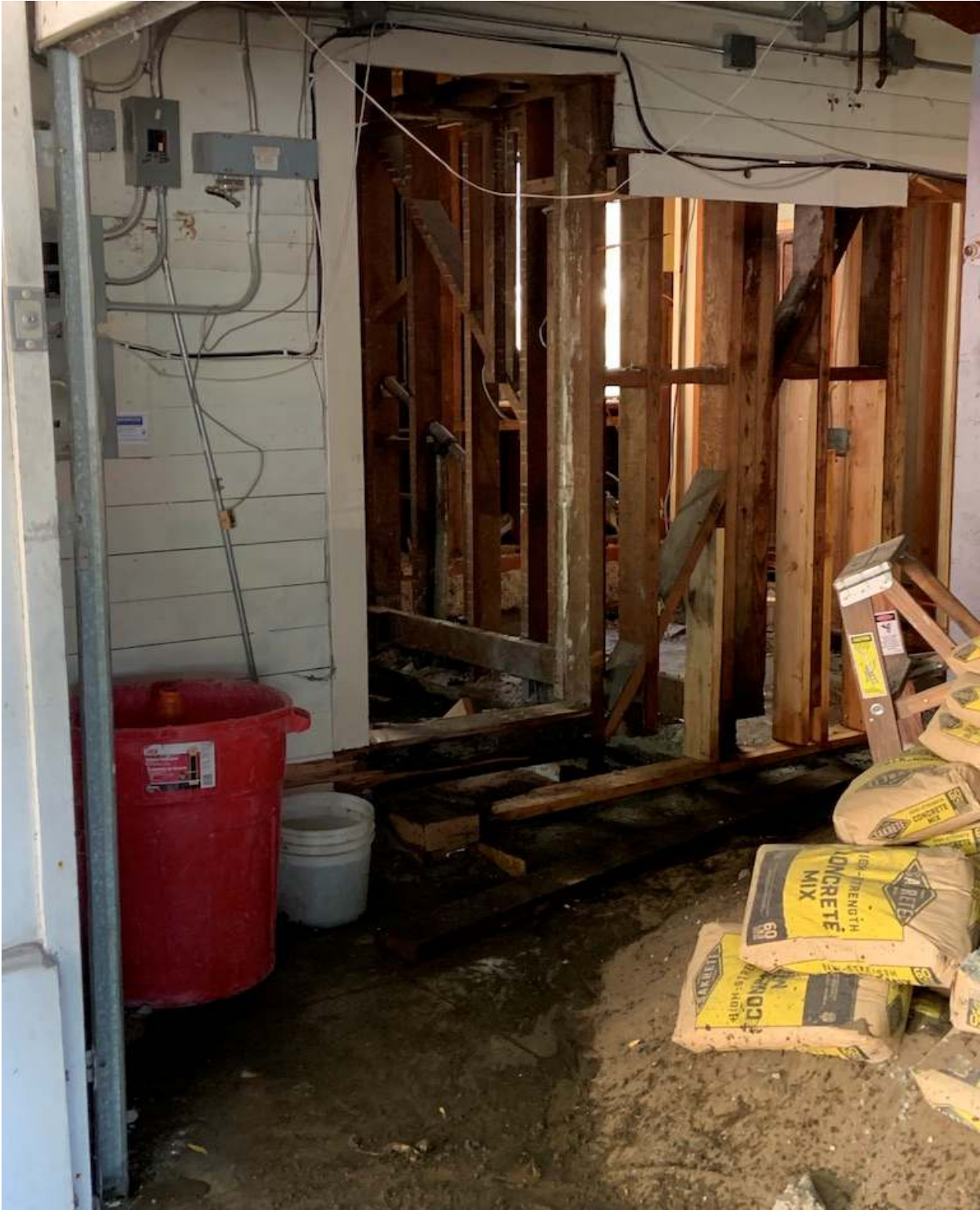
Exhibit 7 ground floor existing bedroom and full bath with former North wall window
