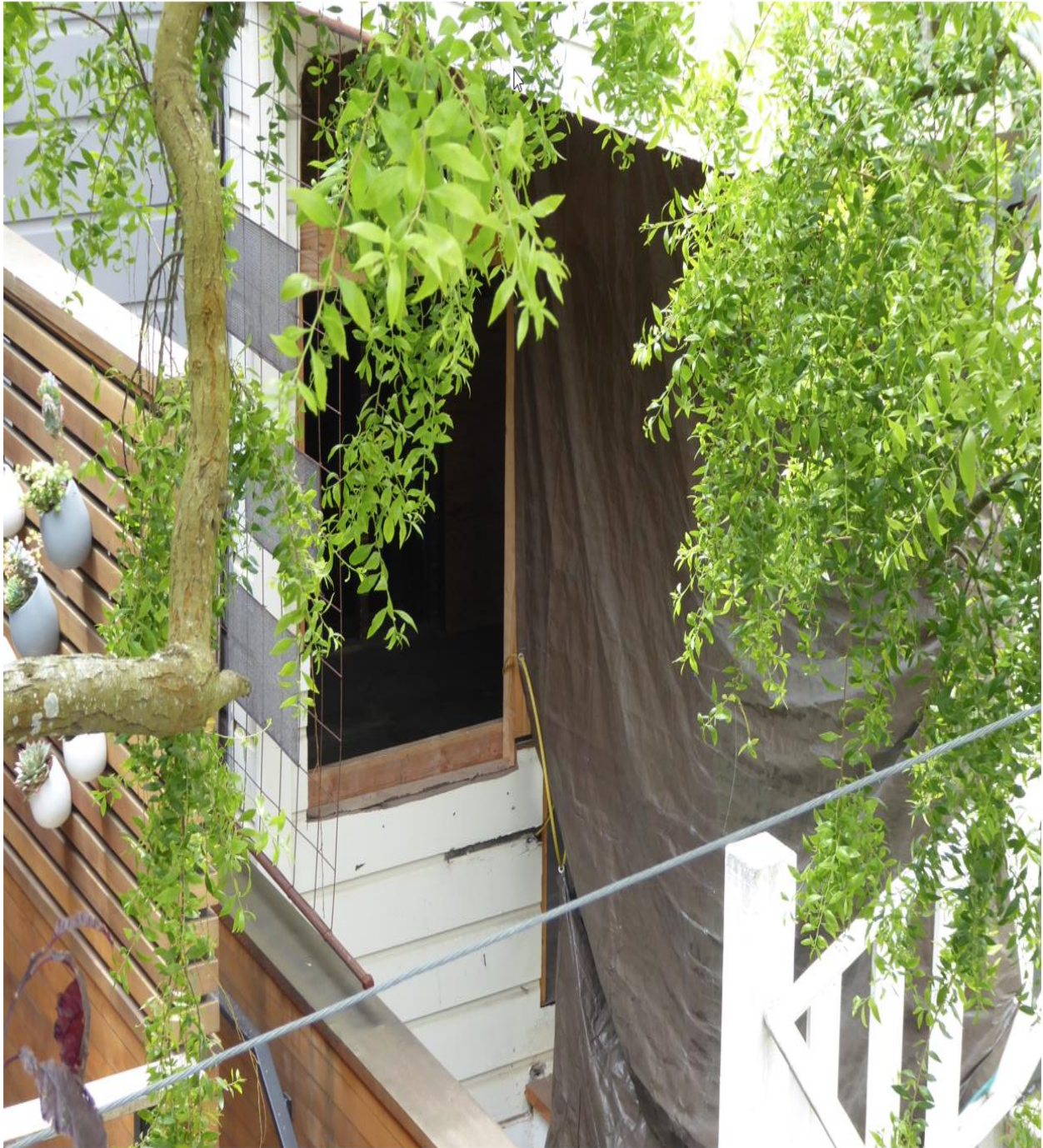
Illegal window removal in former 1 st floor kitchen, no permit.
