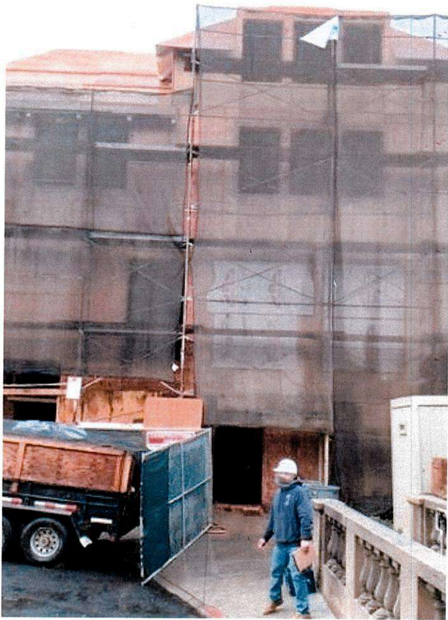
Figure 7 Below Shows the All New Fourth Floor Structure built down the south side of the fourth floor—View Looking Southeast.
