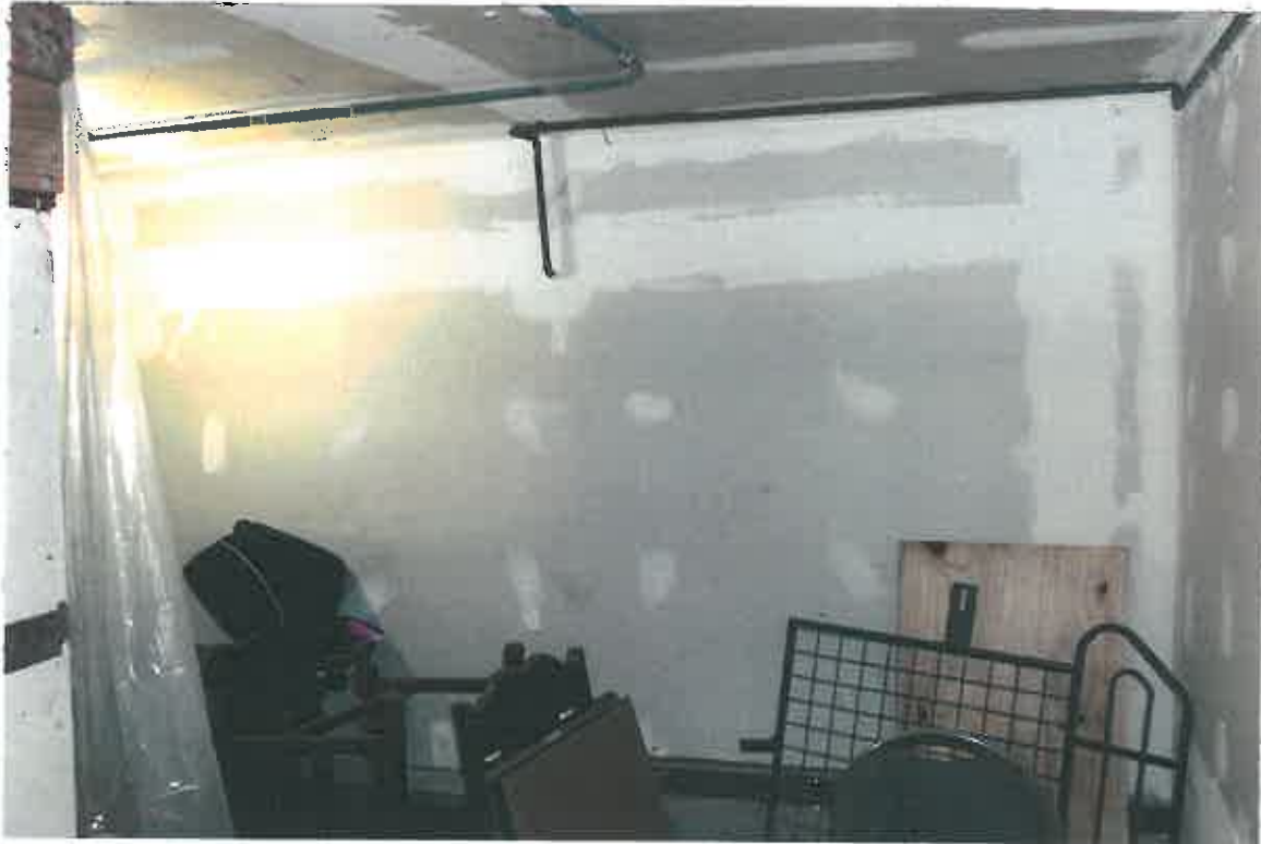
Photo #1, picture of the interior side of one of the shear walls constructed to satisfy San Francisco's Soft-Story Retrofit requirements. Picture taken looking east, in what would be the northern ADU. Note absence of windows.
