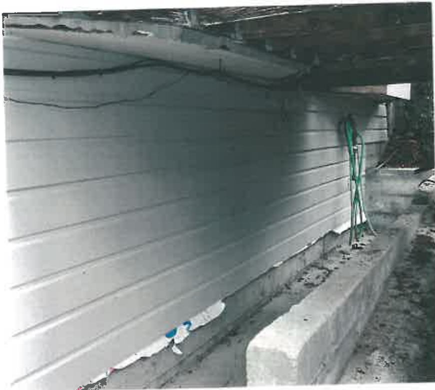
Photo #3, picture of the exterior side of eastern shear wall, and the newly-constructed retaining wall. Picture taken looking north. Note absence of windows.
