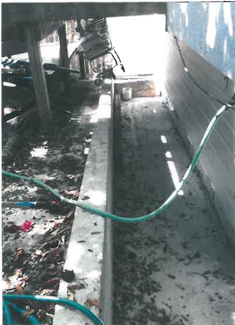
Photo #4, picture of the newly-constructed retaining wall on eastern side of the Building. Picture taken looking south.
