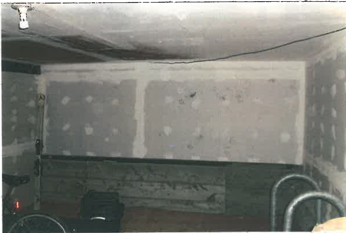
Photo #2, picture of the interior side of one of the shear walls constructed to satisfy San Francisco's Soft-Story Retrofit requirements. Picture taken looking east, in what would be the southern ADU. Note absence of windows.
