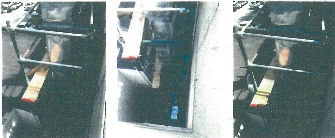
Abatement work consisting of the installation of acoustical duct lagging along the entirety of the mechanical exhaust system's external ductwork.
