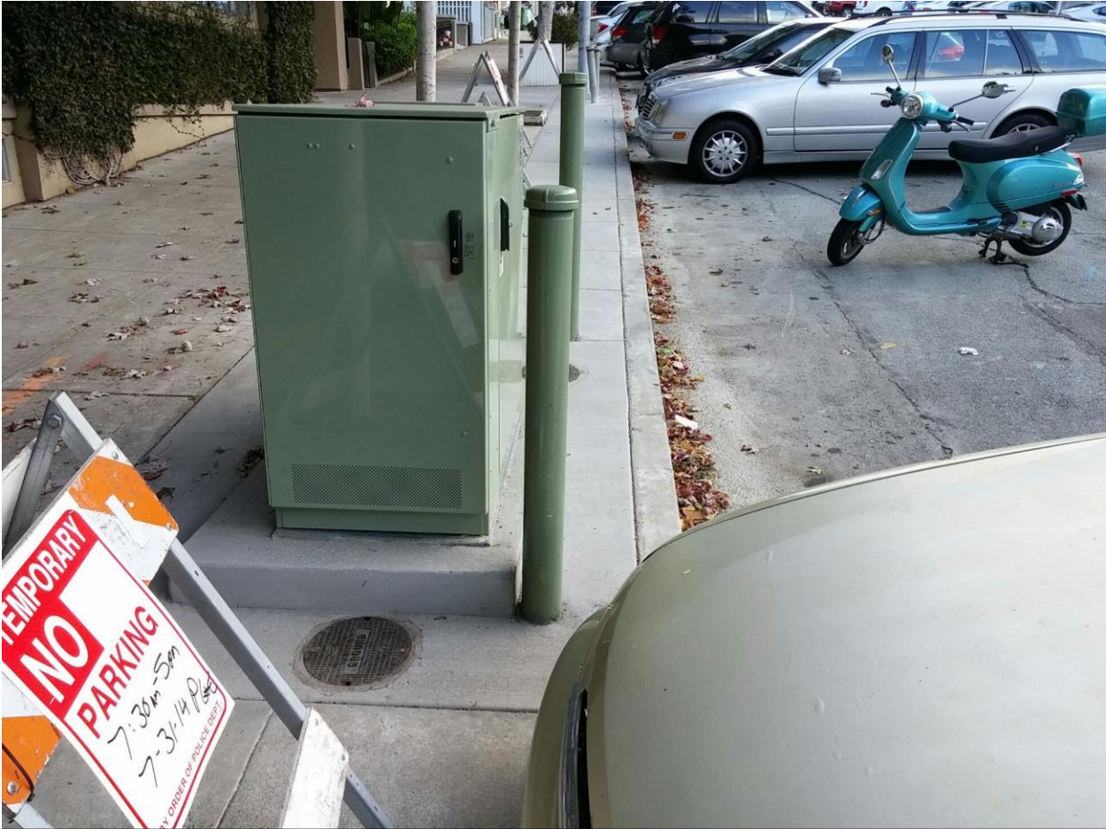
Exhibit D-1: Photo looking north at SMF installed at 698 Pennsylvania Avenue
