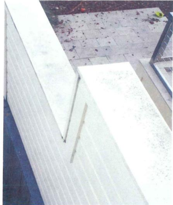
Appellants' high fire wall on their property already provides privacy for decks on both properties.
