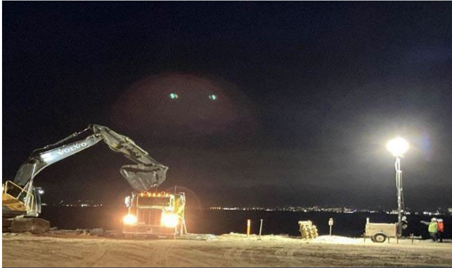
Light towers are used as sun sets to extend excavation activities at IR-03 into the evening
