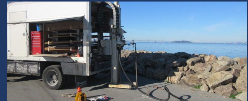
Injection site at IR-26
