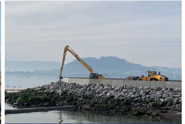
Placement of armor stone on bay side of sea wall (view to southwest)
