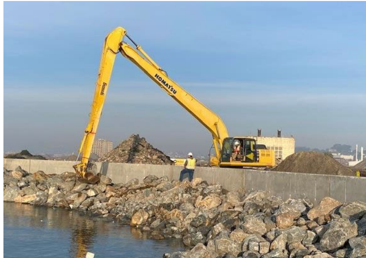
Placement of armor stone on top of filter stone (view to northwest)
