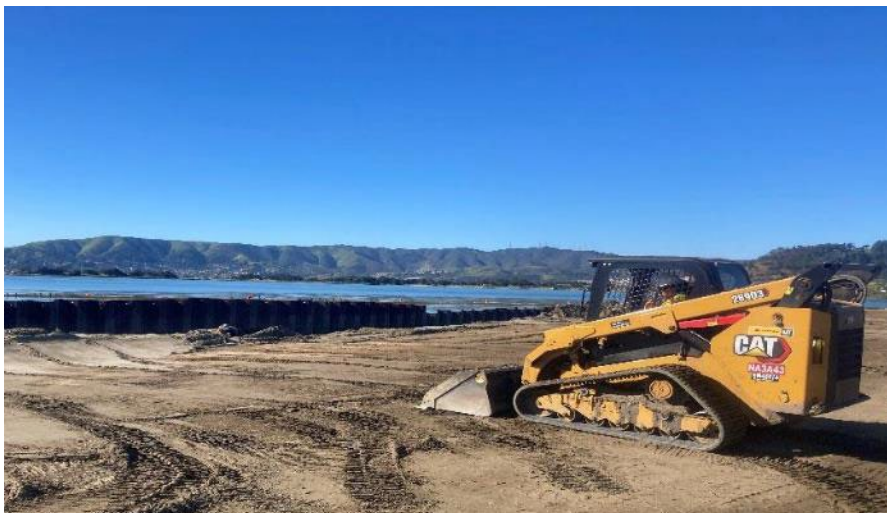
Site grading is part of the preparation for the final solution at the IR-03 shoreline
