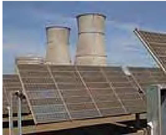
Figure 4-2 - Ground-Mounted PV System
