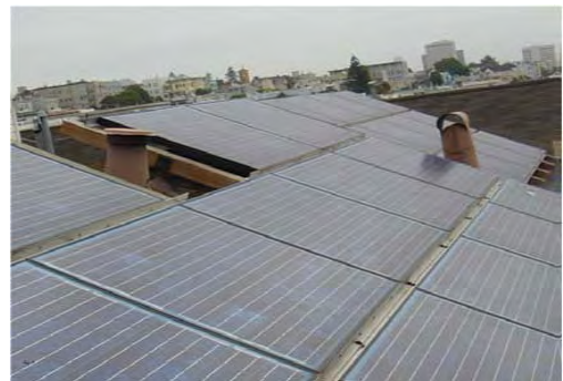
Figure 4-1 - Roof-Mounted Solar System
