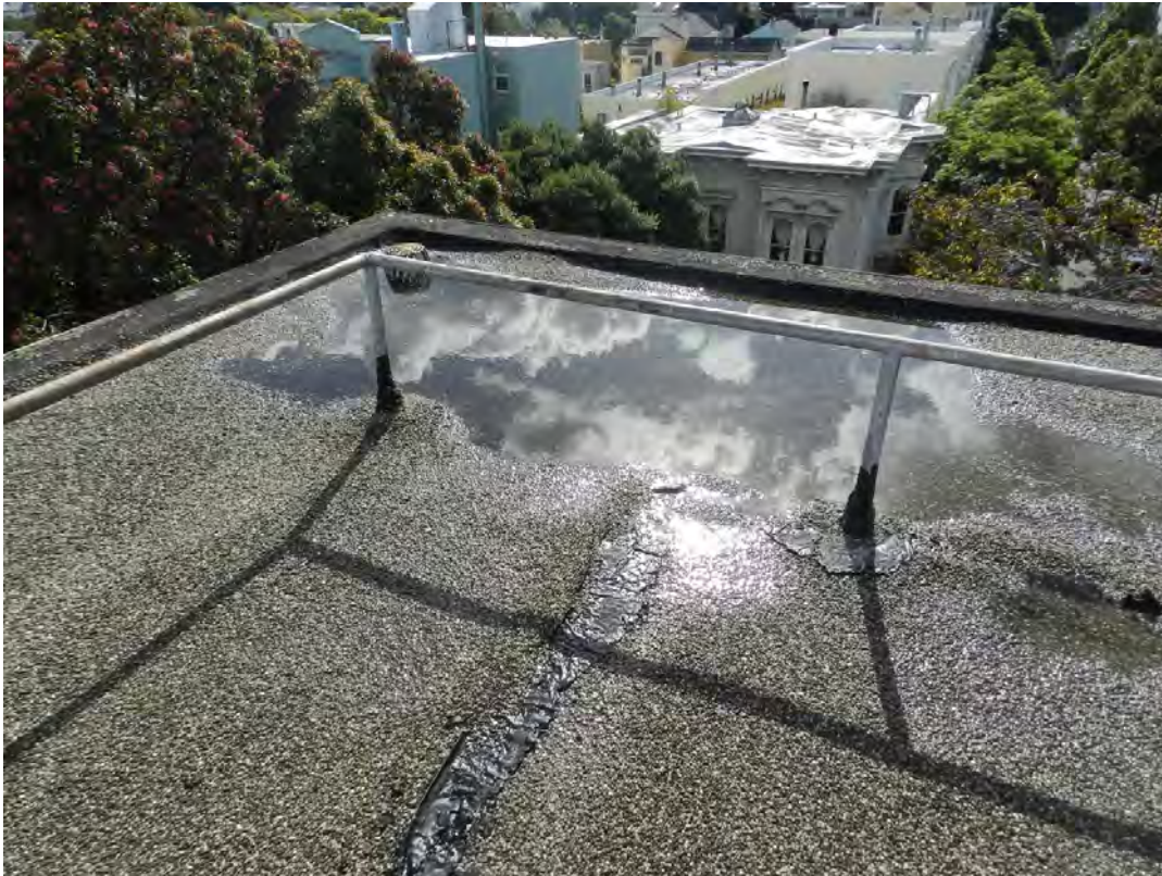
Standing water at 2060 O'Farrell – repairs had been done the day before
