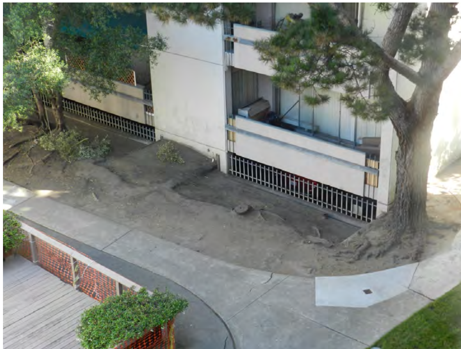
Soils erosion around building 1415 Scott
