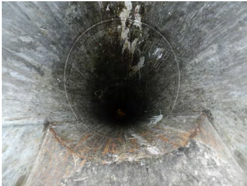
Trash chute at 2060 O'Farrell
