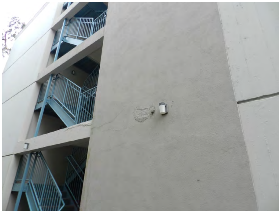
Building mounted lights
