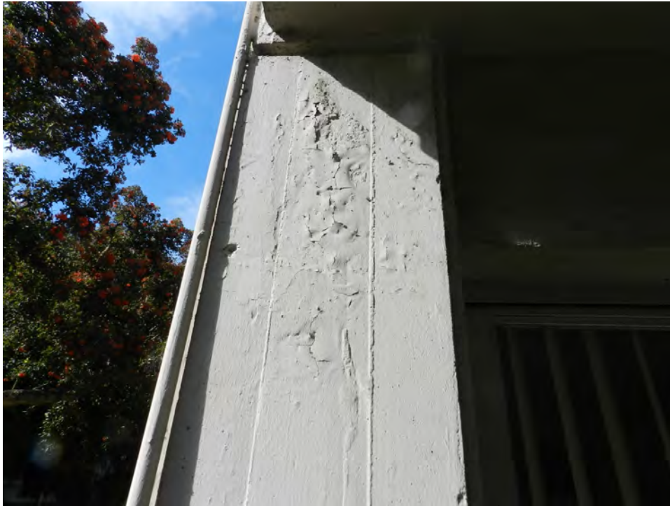
Bubbling paint at exterior wall – 2040 O'Farrell 2 nd floor balcony
