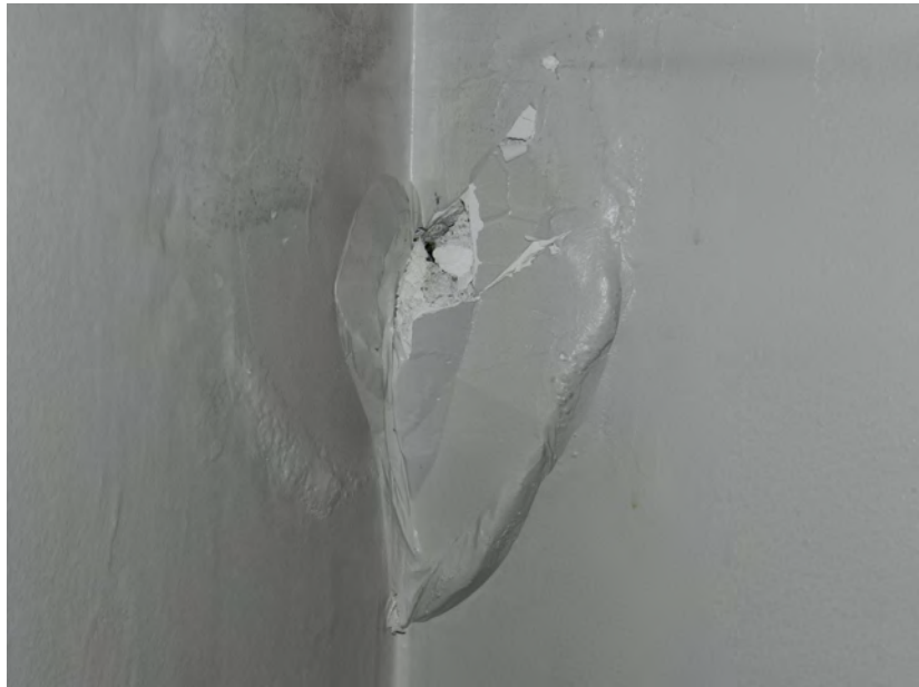
Damage from stair installation at living room of 1 bedroom unit
