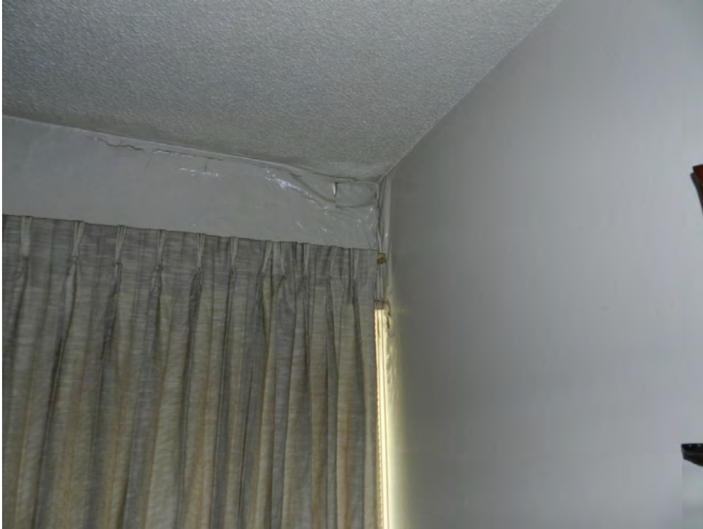
Water penetration into unit – presumably from deck or window above
