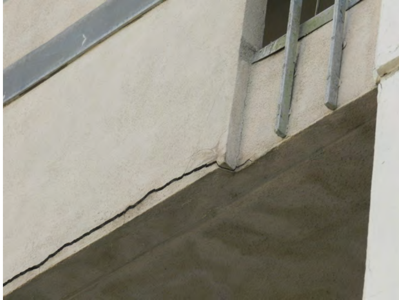
Deck wall detail – separation noted in some locations (this is the 3 rd floor of 1450 Divisadero)
