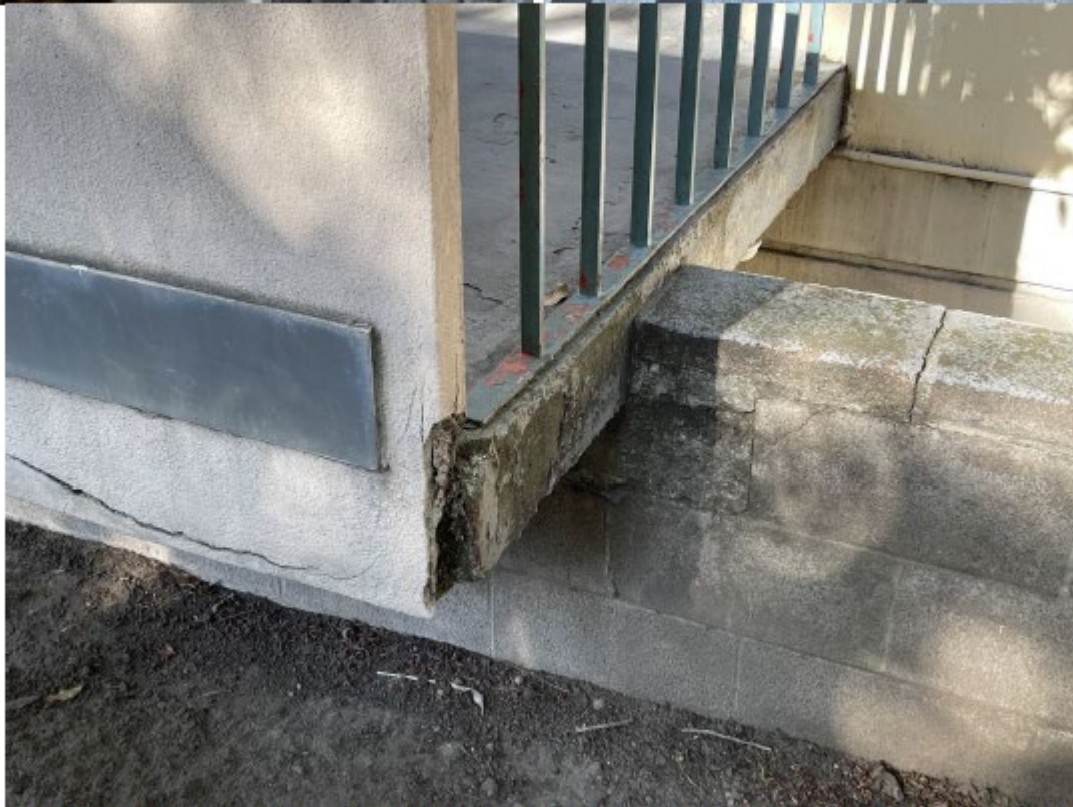
COMMON AREA GUARDRAIL DETERIORATION
