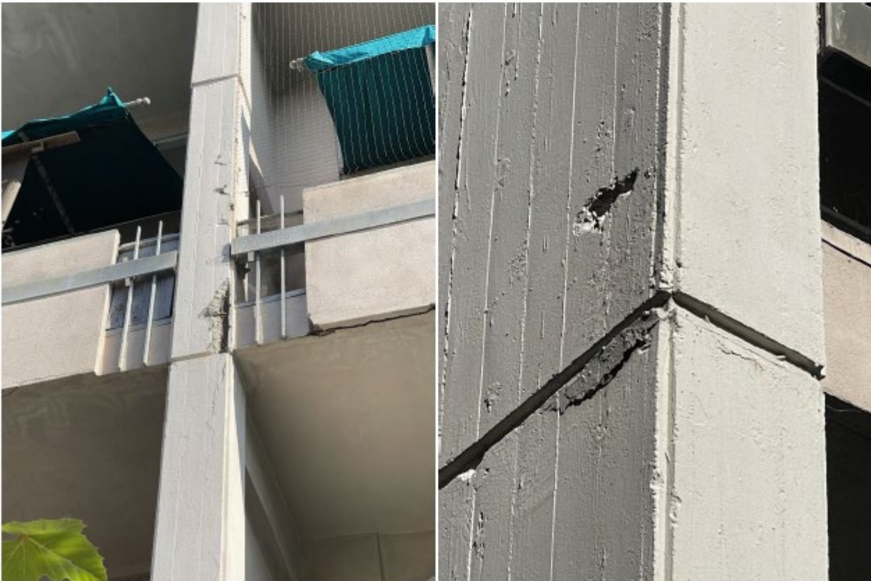
TYPICAL WALL & COLUMN SPALLING
