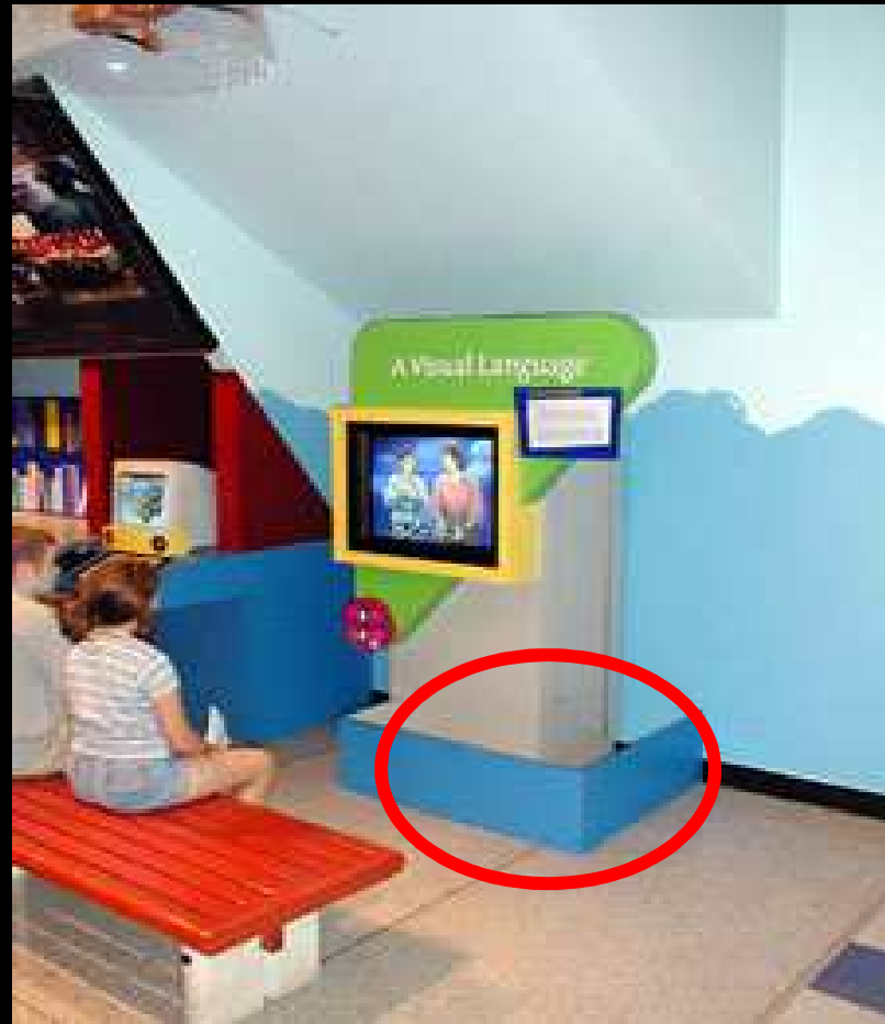
Protruding Object Warning
