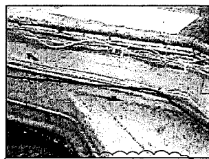
PHOTO 2: EXISTING INTERIOR OF BALCONY, EXISTING ELECTRICAL/TELECOM WIRING & CONDUIT, SEE KEYNOTE 2.42.
