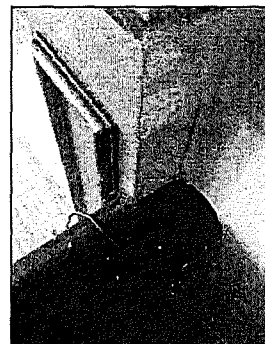
PHOTO 2: HISTORIC HANDRAIL, TO BE SALVAGED AND RETURNED TO OWNERS. USE CAUTION WHEN REMOVING HANDRAIL FROM AROUND PROSCENIUM.
